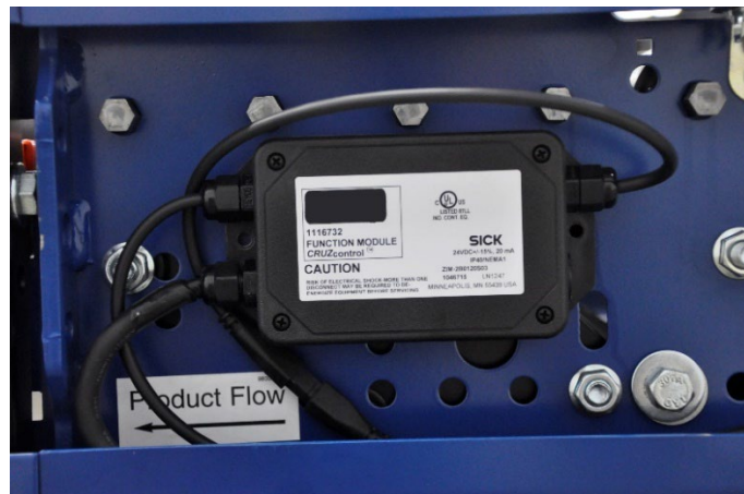
Release function module at discharge end of NBC conveyor. MHS Conveyor part number 1116732.
