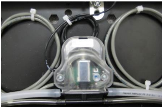
All logic modules lights should be OFF.
